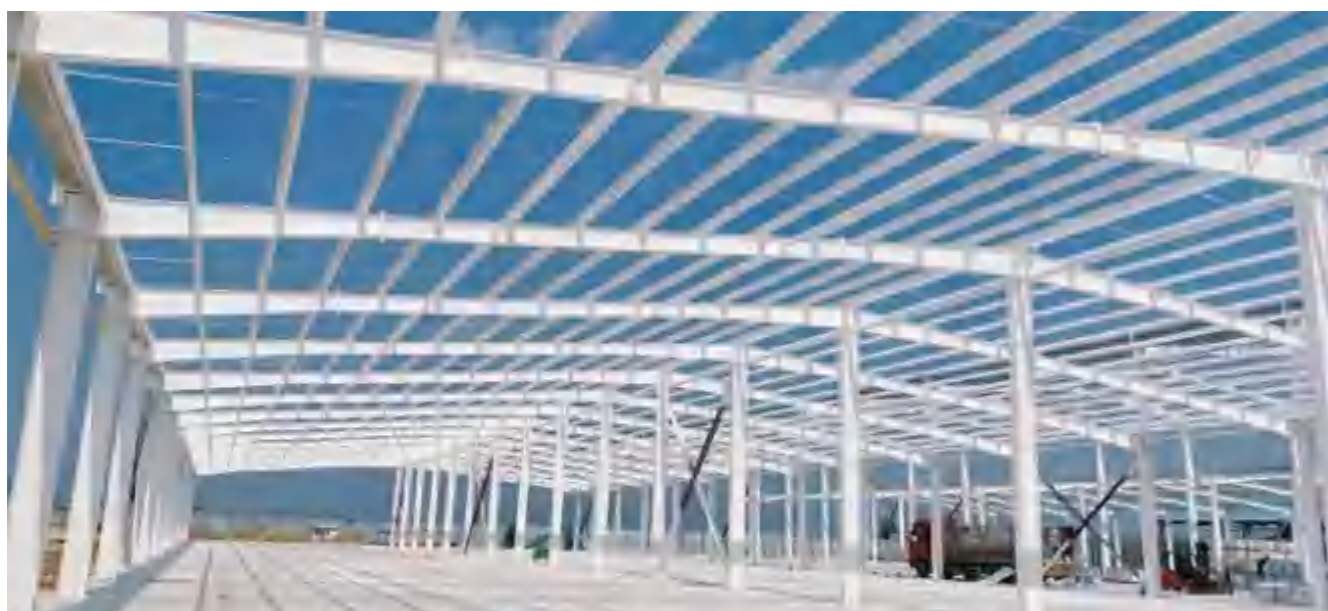
Phase II Project of Yunnan Lesso Technology Development Co., Ltd.
